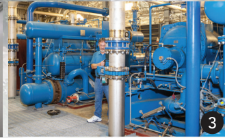
CENTRAL HELIUM LIQUEFIER
